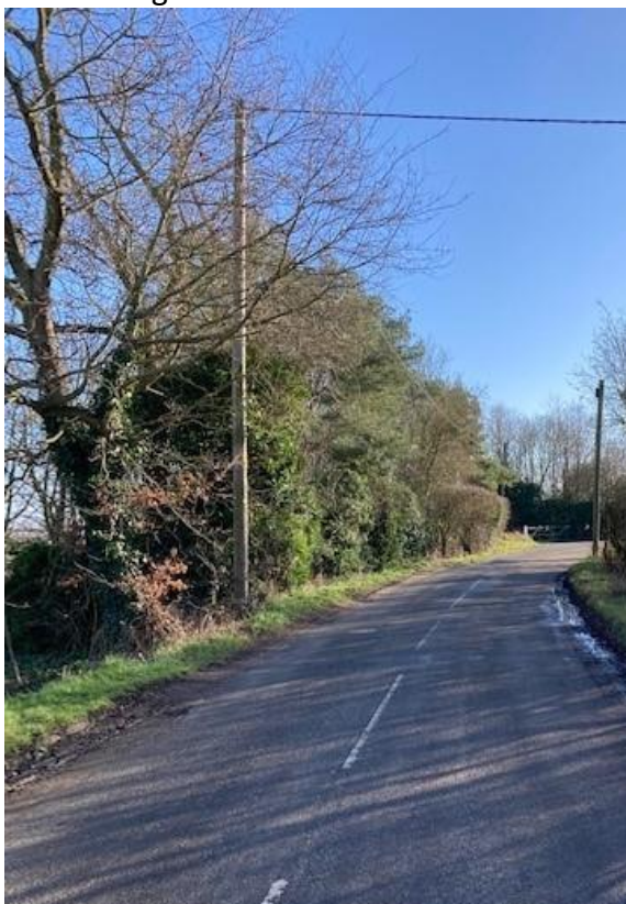
27. Low hanging wires, blind bend, no signage
