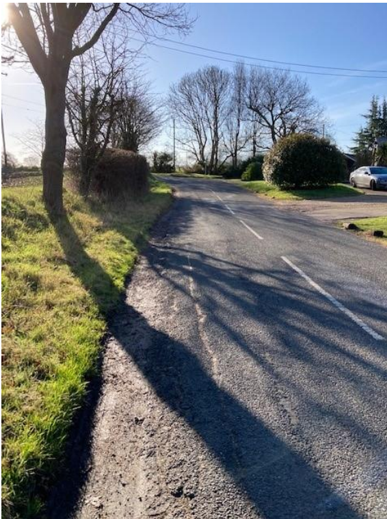
23. Extensive edge of road deterioration and damage
