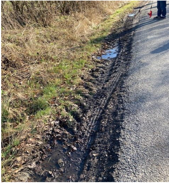
50. To show extensive damage to land and road edge. No safe haven, no passing places and no refuge point for non-vehicle road users
