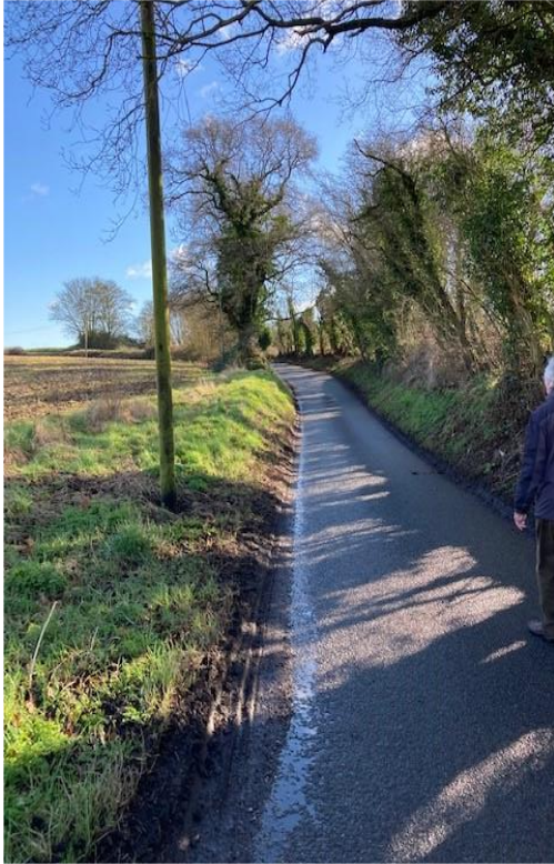
3. Damage to verges and unsighted road
