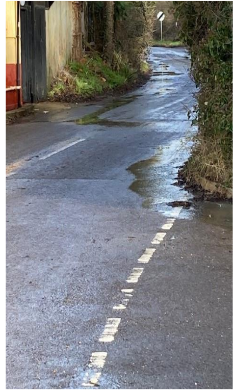
55. Blind junction from B1022 with narrow unsighted lane
