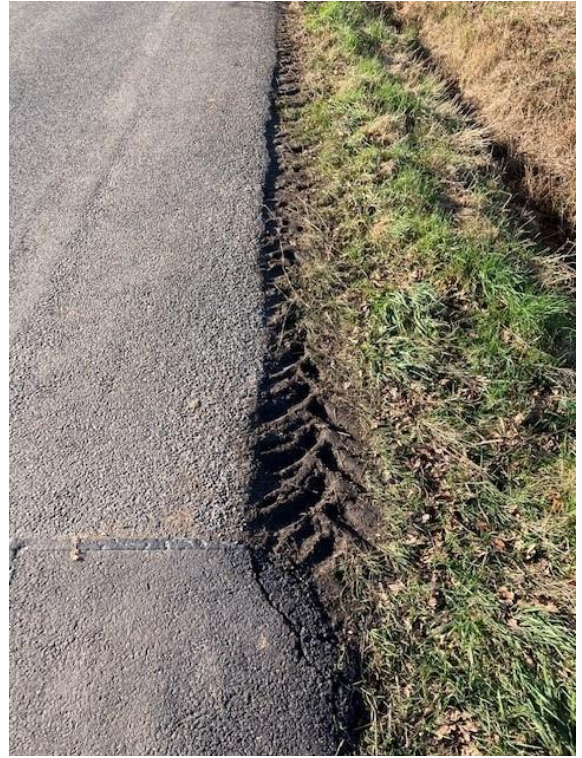
36. To show extensive damage to land as traffic forces a passing place
