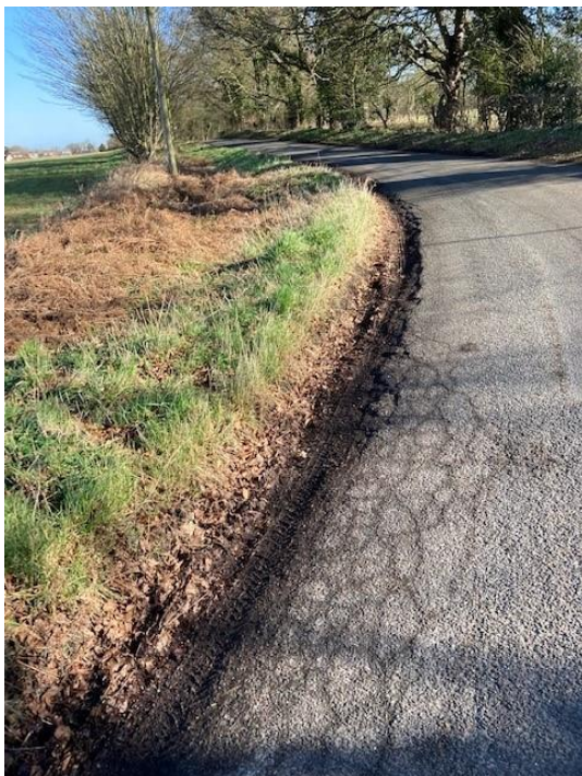
52. Showing erosion and damage to road as traffic forces a passing place
