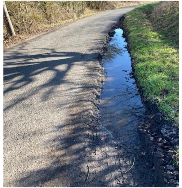
51. Showing extensive road deterioration and damage, no signage warning of school and no safe haven for pedestrians and children
