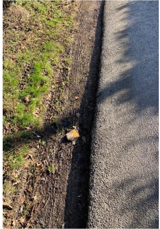
4. Illustrating extensive damage and destruction to verges and edges
